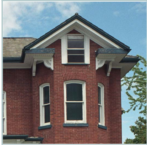
There are brackets under the returned eaves of the gable on the southeast projecting bay but they are missing from the west bay.
