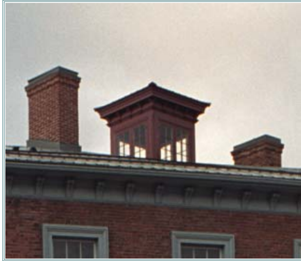
The rooftop lantern had been removed and has now been restored. The Great Farini began a daring high wire walk across the Ganaraska River starting at the lantern of the Waddell Block in May 1861.
