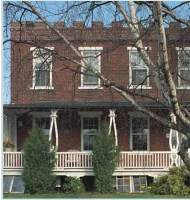
The battlemented parapet, six over six double-hung sash windows, door case with sidelights and transom, and trellised verandah with lyre-shaped supports are all original details.
